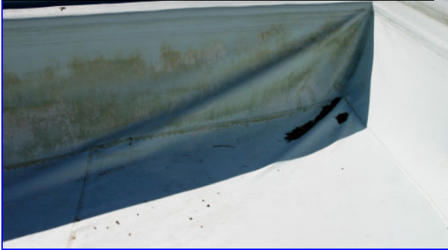
Folds & Discoloration Across the PVC Liner
