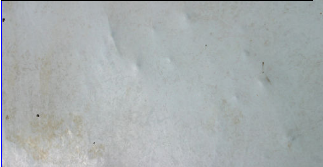
Chunks of Broken Concrete Evident Under the PVC Liner
