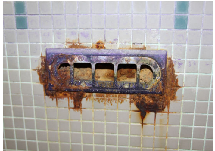
Corroded, Rust filled, Manganese covered return line
