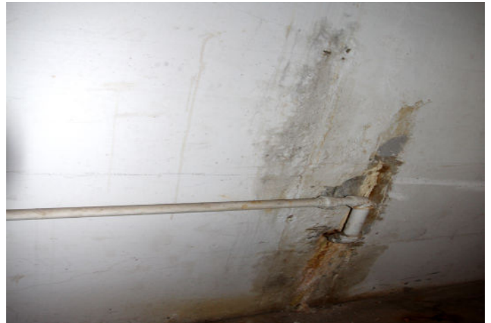
Calcium leaching from wall & around steel piping
