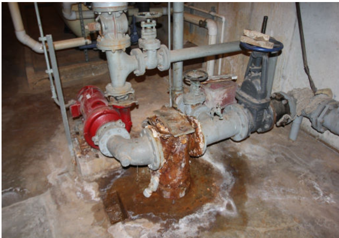
Condition of Strainer Before Renovation
