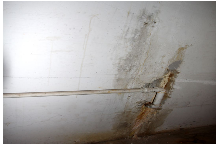
Calcium leaching from wall & around steel piping
