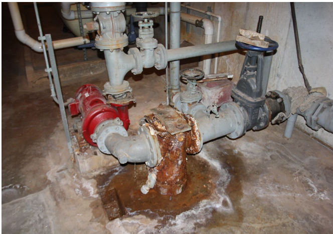
Condition of Strainer Before Renovation
