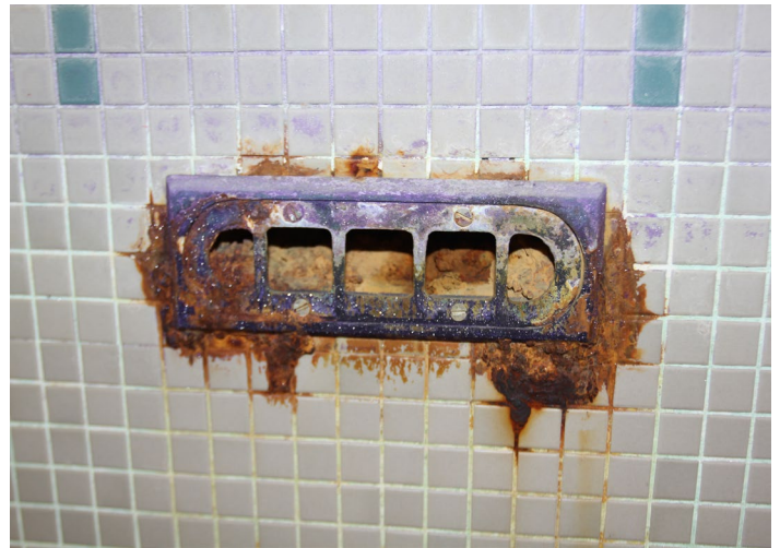
Corroded, Rust filled, Manganese covered return line
